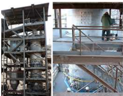
Fig. 1 Shaft furnace for magnesite sintering-general view
